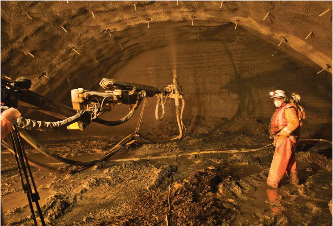
The Sika Aliva PM500 robotic arm sprays the shotcrete containing Sika ViscoCrete SC305 retarding superplasticiser, and Sigunit L53-AF accelerator for sprayed concrete
