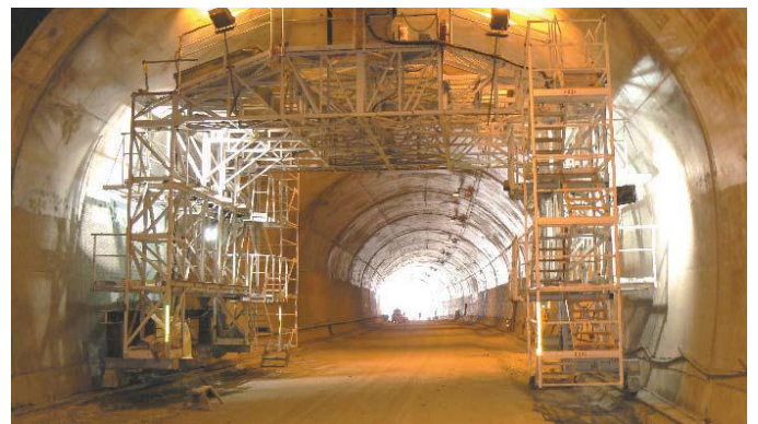
The concrete tunnel lining was then poured against the Sikaplan membrane. The concrete contained Sika ViscoCrete 5-500 a superplasticiser for an ultra-smooth finish.
